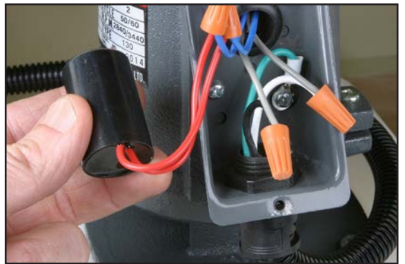
Figure 50. Pump motor wiring and capacitor (M2).
