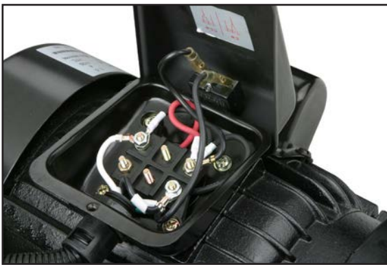
Figure 48. Junction box (M1).
