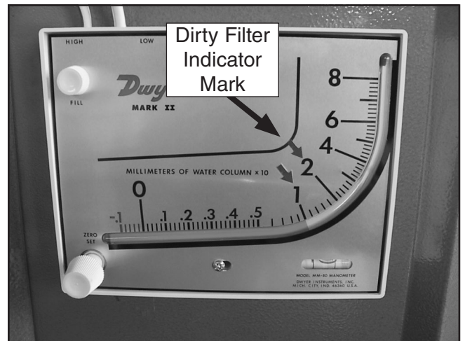
Figure 29. Dirty filter mark example.
